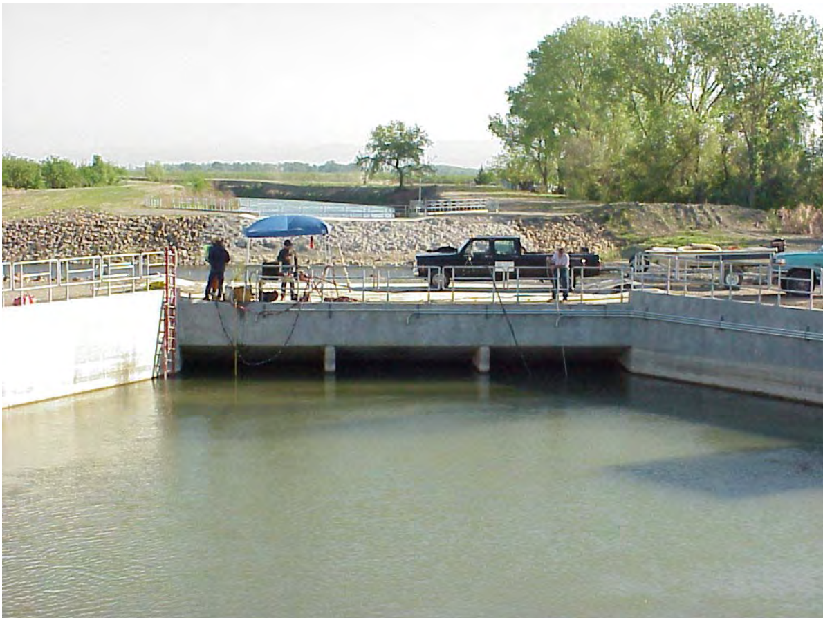
Figure 2. The Stony Creek Siphon channels, looking upstream towards the effluent end of the siphon.
