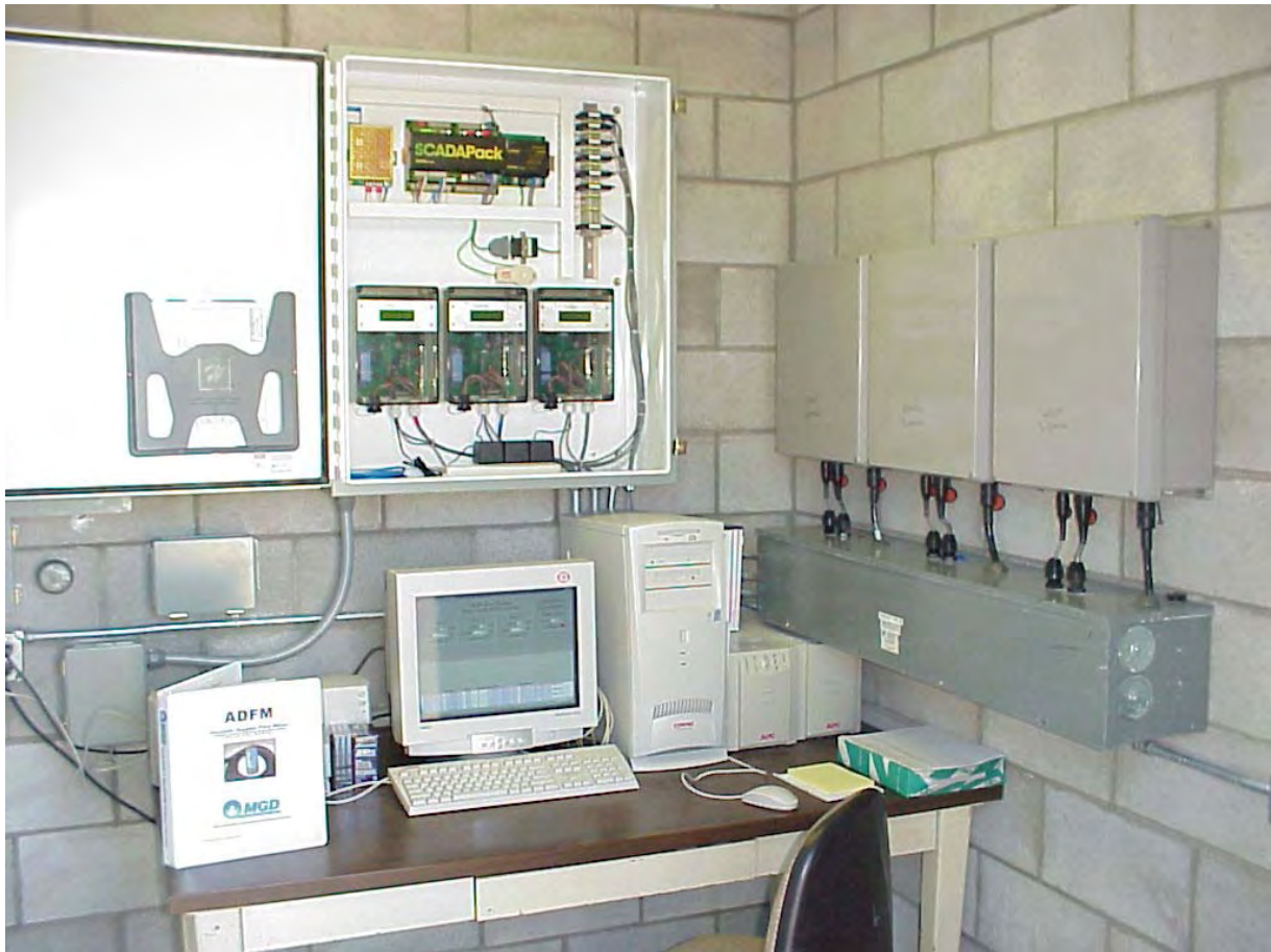
Figure 5. Electronics installation in the gauge house. This system provides real-time output of the data.
